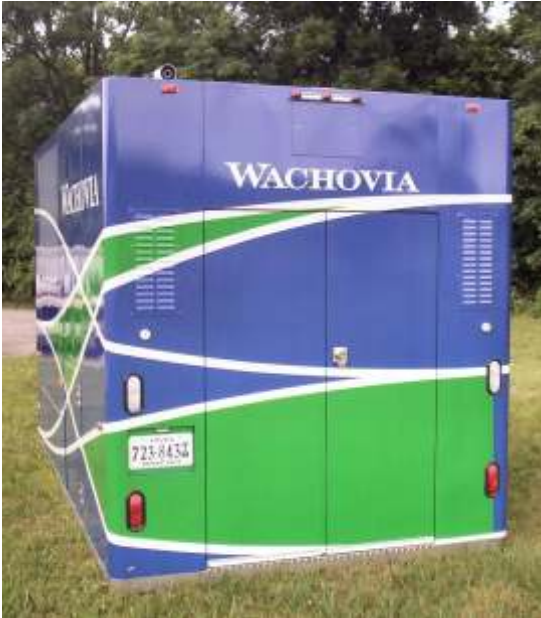
View of the Propane Generator access doors.
