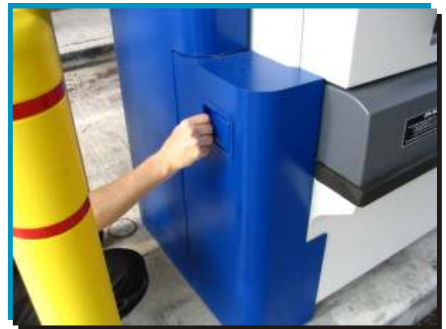
Security Panels Lock Into Place; Keyed Access Allows Easy Unlocking for Service Personnel
